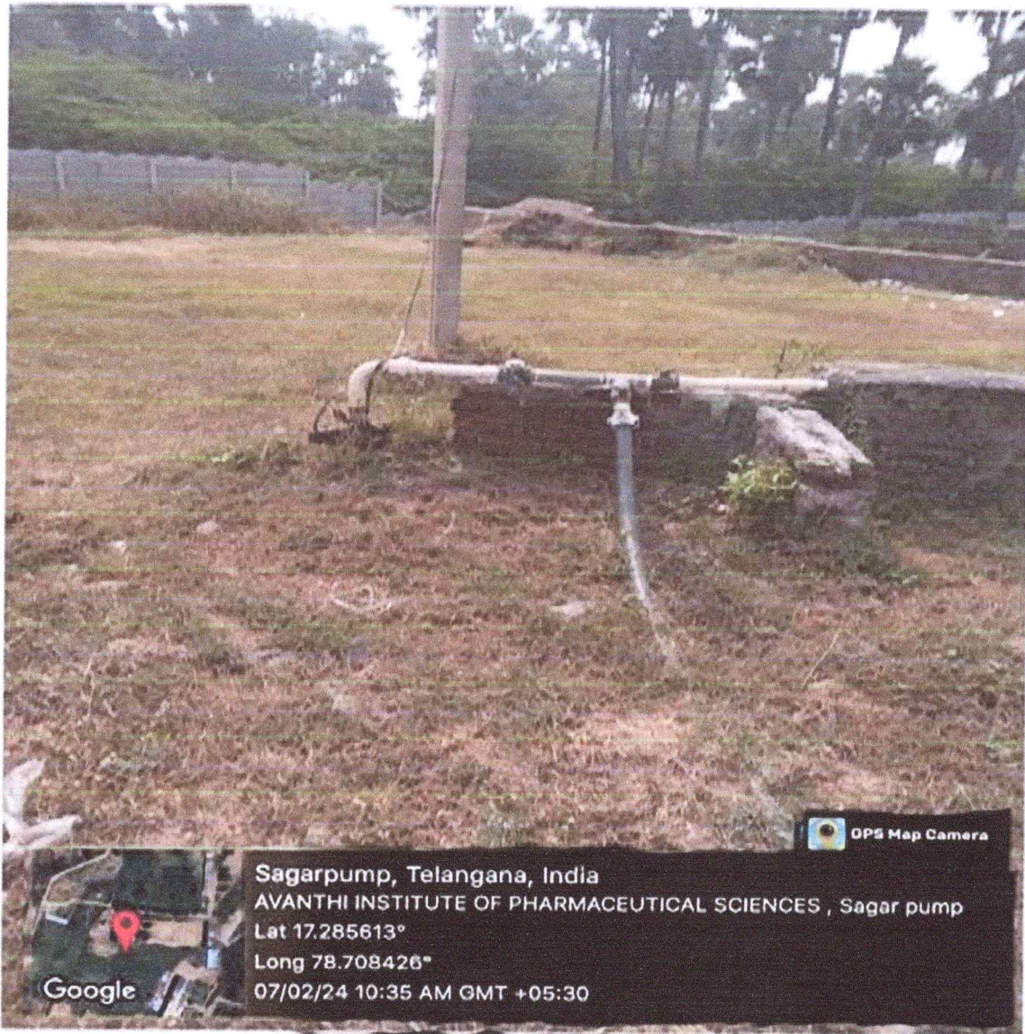
7HP Motor capacity was installed opposite to girls hostel
