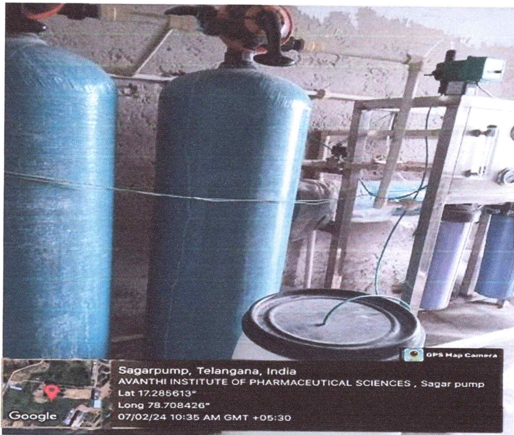
RO plant purified water Plant
